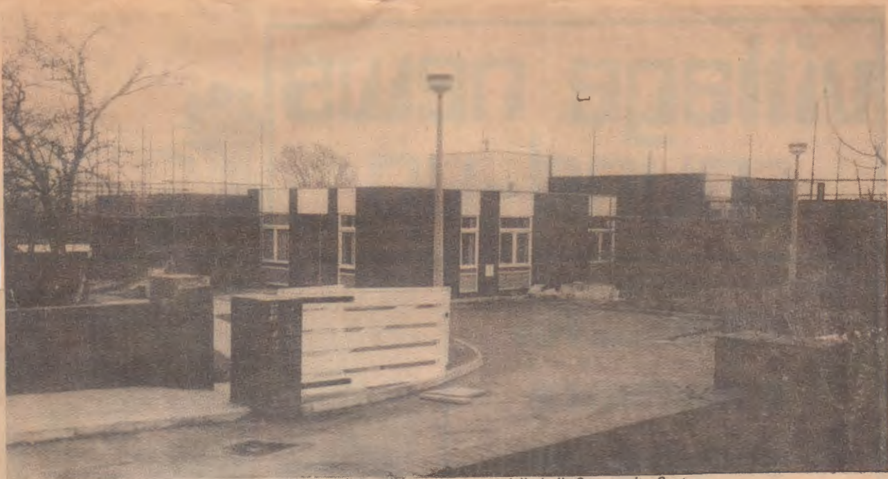
Hathern Junior School and, to the left, the partially built Community Centre.
